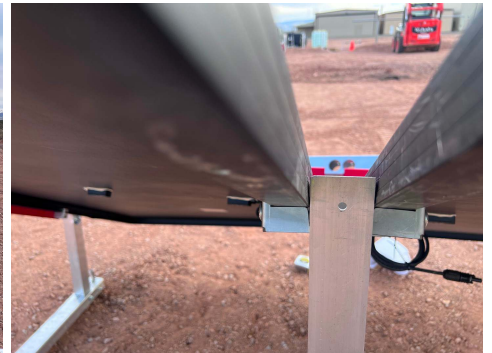
PHOTO 12: Middle brackets after testing
